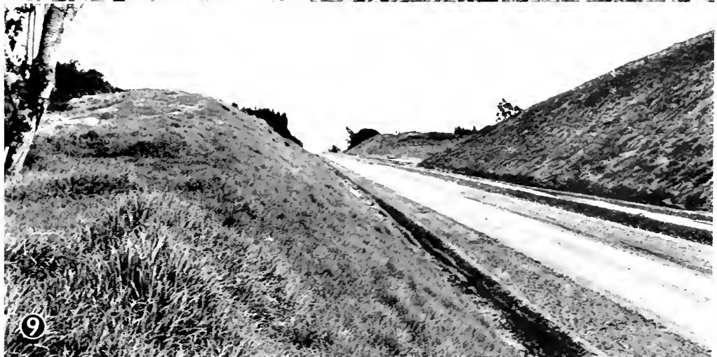
Typical erosion occurring on cut slopes during construction are shown in Nos. 7 and 8. On the same job and same soil 1\frac{1}{2} :1 cut slopes are shown in No. 9 that were stabilized with top soil, rye grass and straw
